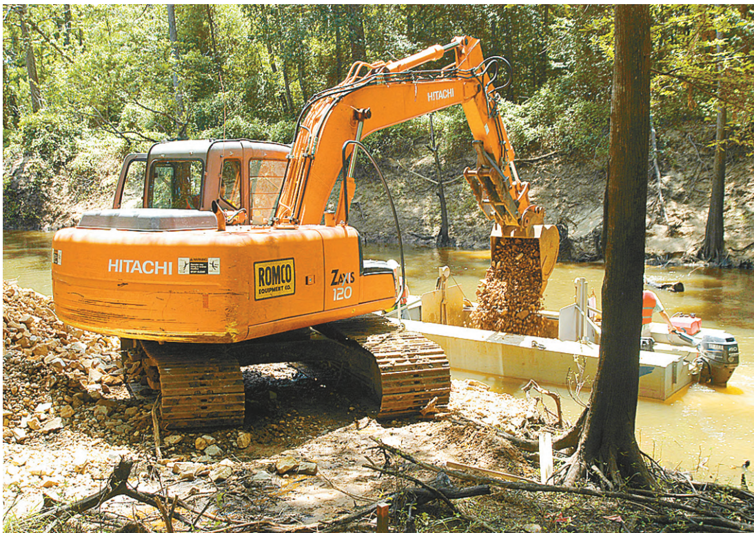
THE EFFORT to re-create the spawning grounds of the native paddlefish in Big Cypress Bayou included the placement of special rocks along the bottom of the stream. The rocks were loaded into a specially built boat by a Kilgore firm before they were carried downstream and deposited in the proper location.
